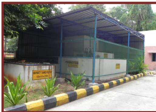
WASTE WATER TREATMENT PLANT
